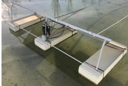
Fig. 3 Inverter on floating modules ( Source: CEDER CIEMAT )
