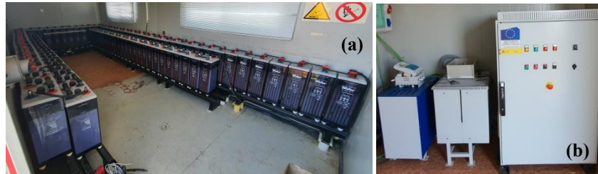
Fig. 5 (a) Lead-acid batteries Fig.5 (b) DC/AC inverter. Note: Own source.
