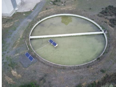
Fig. 1 Aerial view of the floating photovoltaic installation (Source: CEDER CIEMAT)
