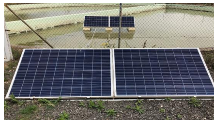
Fig. 2 Photovoltaic modules ground and water (Source: CEDER CIEMAT)
